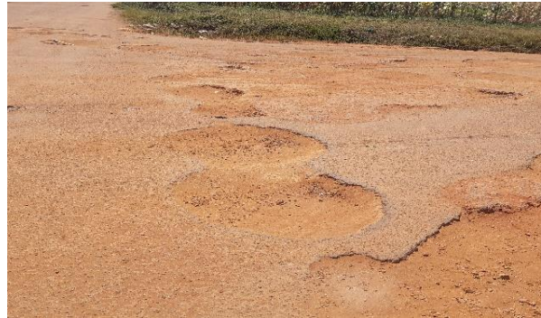
Potholes along Market Road
